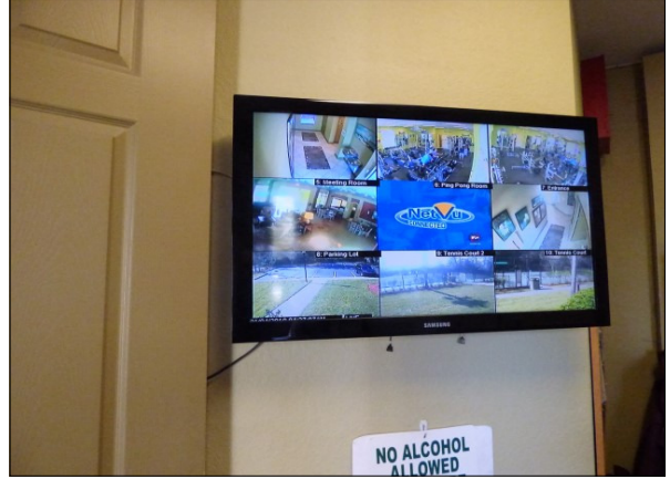
Security Camera System
